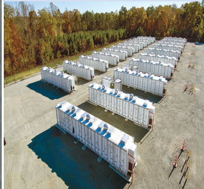
An electricity storage facility near Topping would resemble this one owned by Dominion Energy. Each container stores 8 MWh. (Photo courtesy of Dominion Energy)
