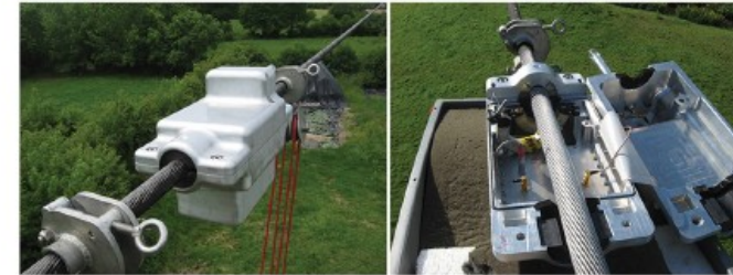
The completed installation of an Ampacimon real-time sensor on a transmission line conductor and a look at the inside of the sensor.
