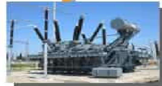
Phase Shifting Xfmrs - Regulate phase angle (δ), limited by MVA, angular range
